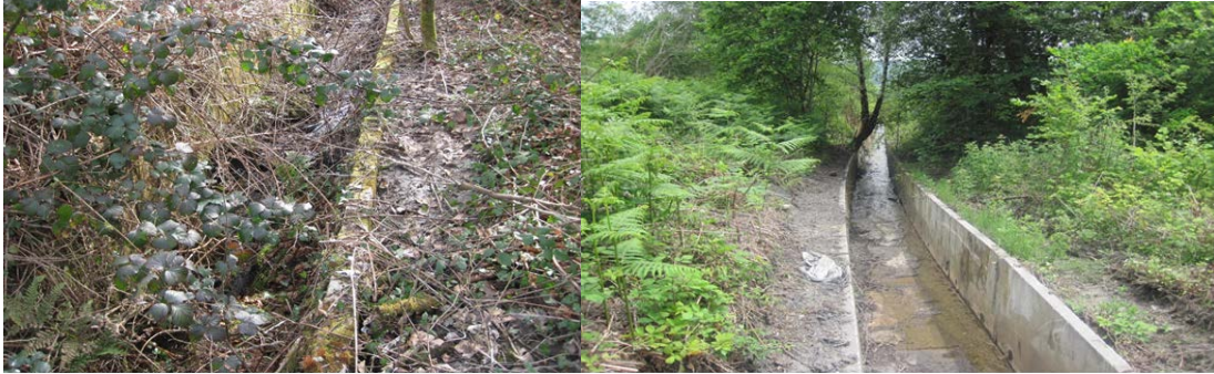
Site photographs taken on site to demonstrate the effective clearance of a tip concrete drainage channel
